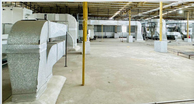
Ducting with M S Angle frames...
