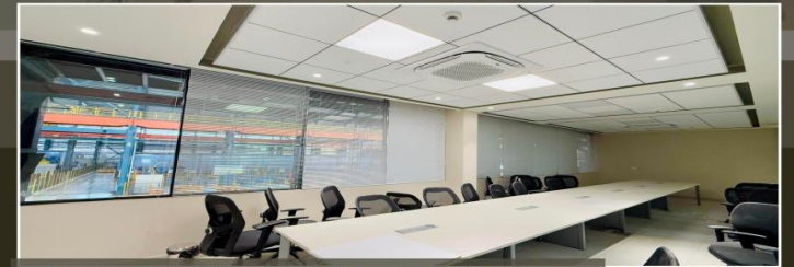
Our Recent Project of Carrier VRF @ TATA Steel Downstream Products LTD
