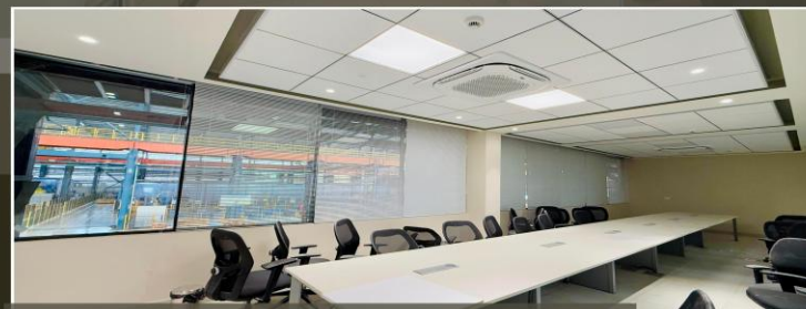
Our Recent Project of Carrier VRF @ TATA Steel Downstream Products LTD
